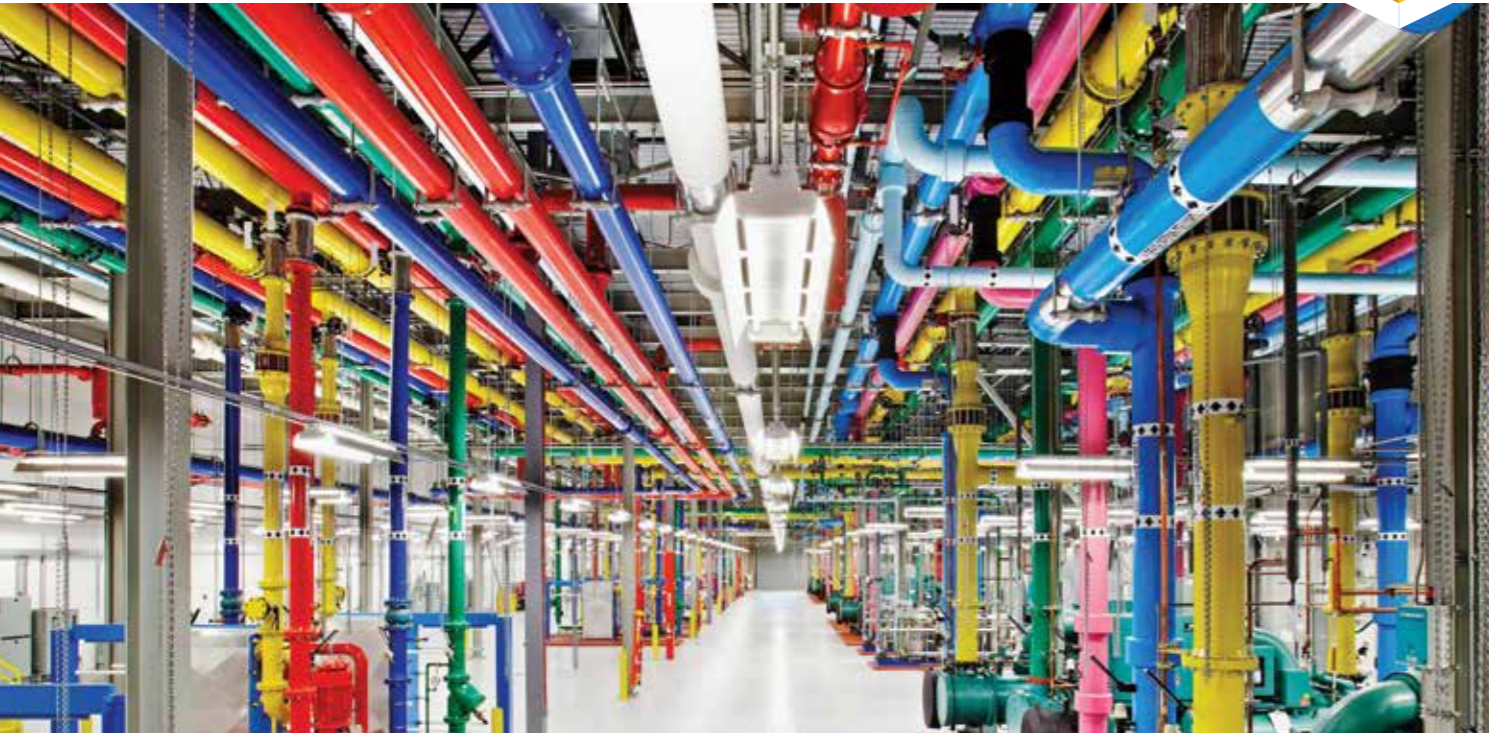
Above: A central cooling plant in Google's data centre in Georgia, USA. Previous page: Professor Paul Bonnington in the Monash CAVE2™, which is used to visualise big data. (CAVE2 is a trademark of the University of Illinois Board of Trustees). Image: Paul Jones, Coretext.
